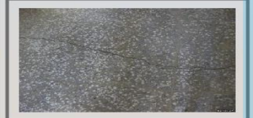
Floor tile dam aged during track installation
