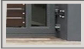
Unaligned of track and floor level cause awful appearance
