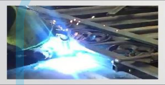
Welding process will defect the finishing
